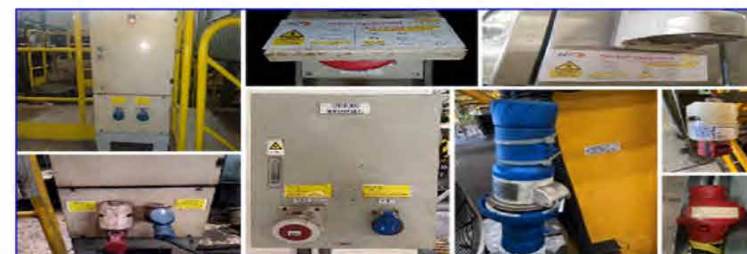
Some outlet of electric equipment was displayed
